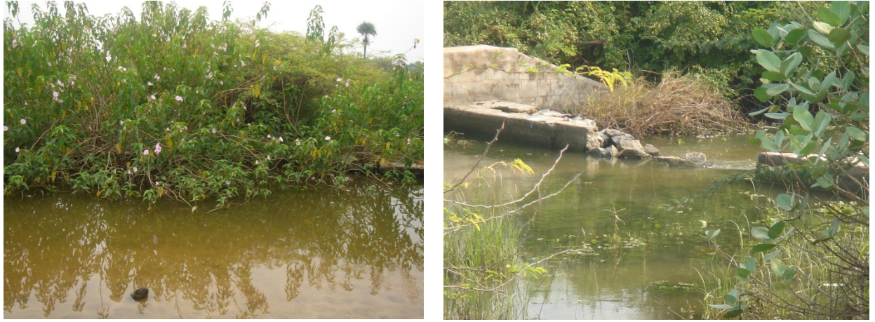
Figure 2. Check dams encroached by bushes (left) and damaged by people (right) at Dabbidikunta watershed
