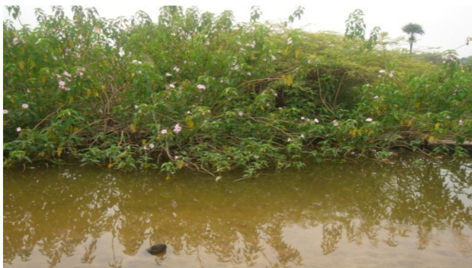
Fig: Check dam full of bushes around head wall needs cleaning
