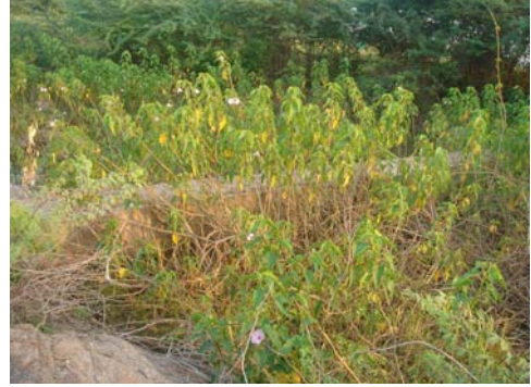
Check dams needs repair and cleaning and desilting for better
