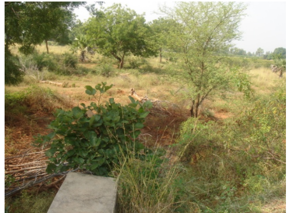
Repair, cleaning and desilting is required for this check dam
