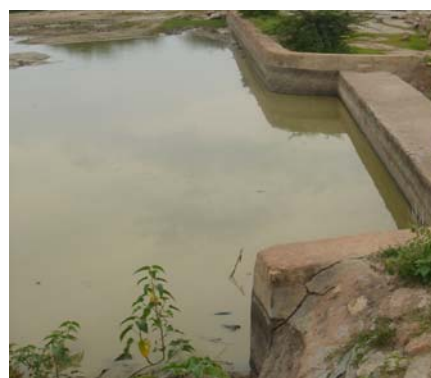
Fig; Check Dam constructed near Md Mohan's field improved water availability in his well
