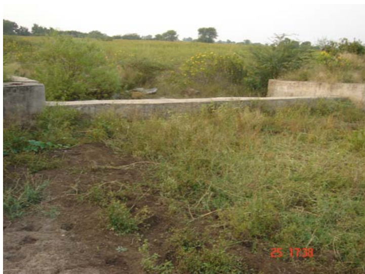
Fig: Check dam silted up need to be cleared for proper functioning.
