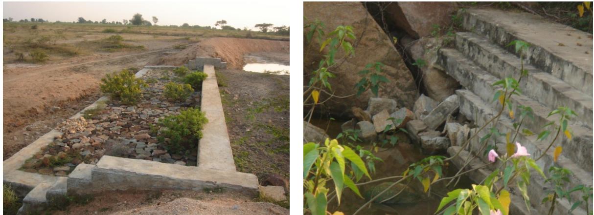
Figure 3. PT filled with sediment (left) and CD developed leakages (right), Pragathi watershed
