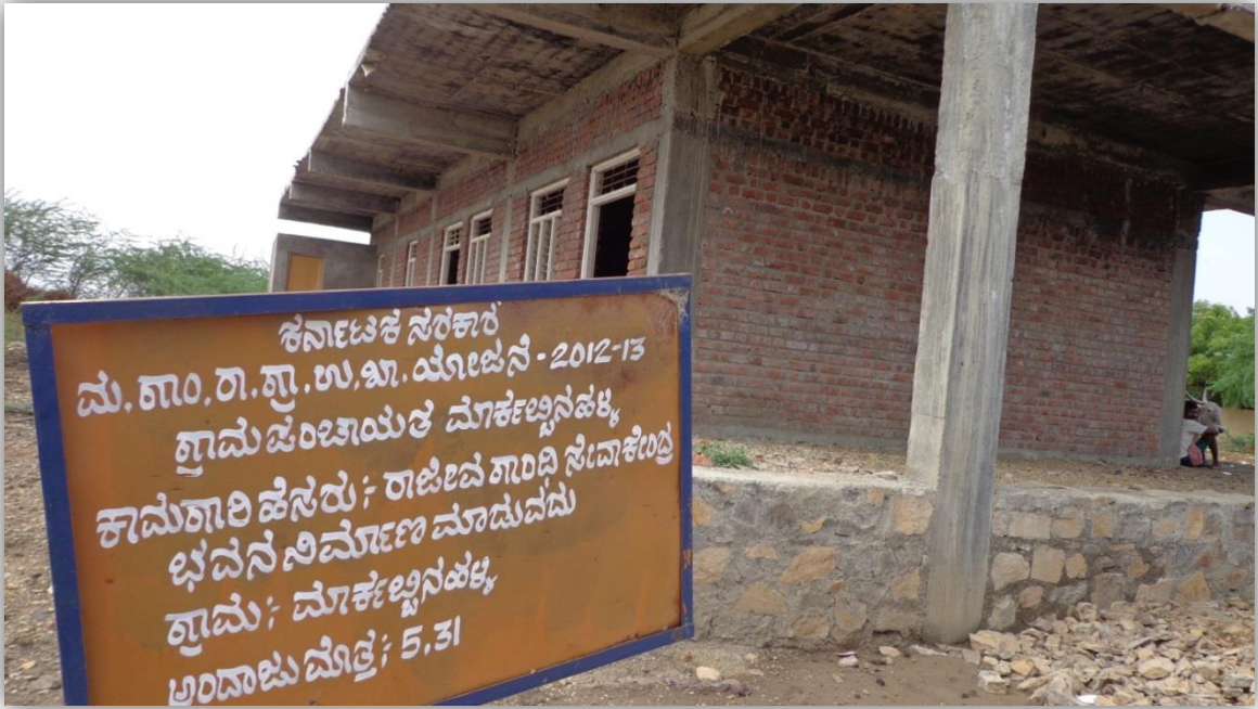
Plate 1: Rajiv Gandhi Seva Kendra under construction as part of MGNREGP in Markabbinahalli village. [Dated 10-05-2013]
