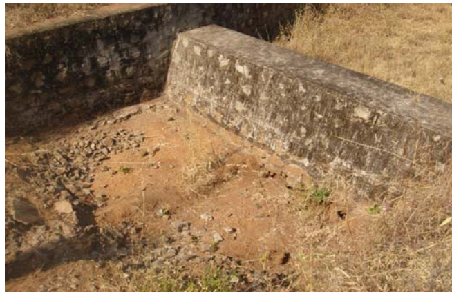
Figure 2. Damage of apron wall at Neredavai watershed, Mothey Mandal
