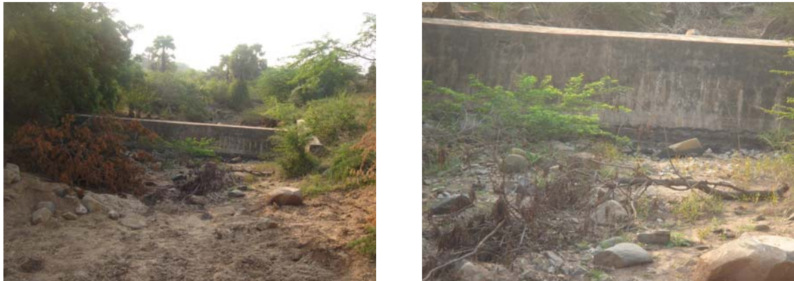
Figure 1. Masonry check dam (left) and damaged apron wall with leakages (right) at Karshak watershed, Akaram village, Shaligouraram Mandal
