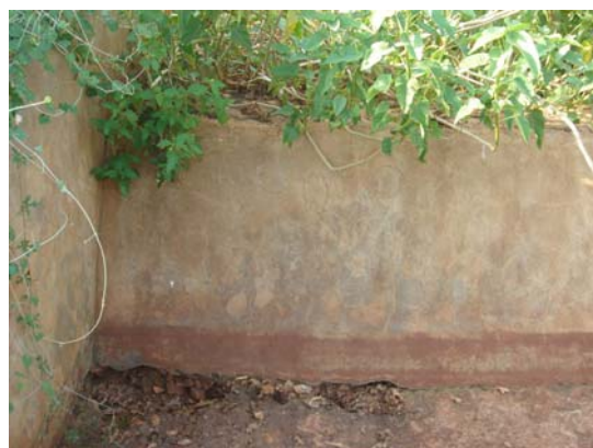
Figure 2. Leakage from check dam at Yerrakunta watershed, Shaligouraram Mandal
