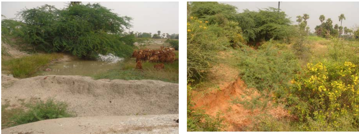
Figure 2. Poor maintenance of the structures at Bairavudu watershed, Shaligouraram Mandal
