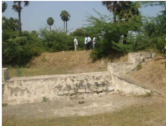
Figure 2. Leakages from check dam at Peddacheruvu watershed, Shaligouraram Mandal
