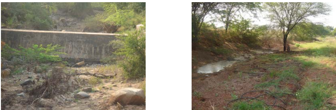
Figure 2. Poor maintenance of the structures at Hanuman watershed, Mothey Mandal
