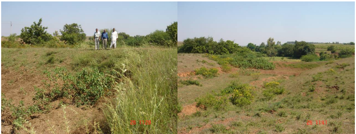
Fig: Percolation tank benefitting for lot of percolation of water with lot of silt deposition and shrubs needs removal
