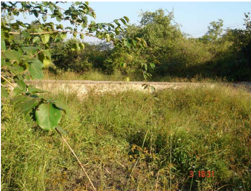
Fig: Check dam benefitting 40 acre farmers' fields is silted up and a big hole at corner of CD having no storage of water needs repair.
