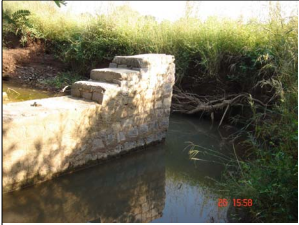
Picture 9. Breached away check dam in Edulapally watershed.
