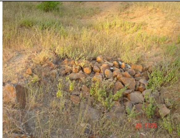
Picture 6. Damaged loose boulder structure in Budera watershed.
