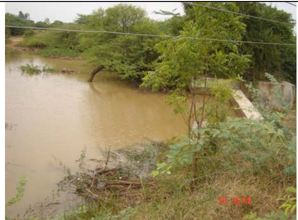
Picture 24. Masonry check dam in the Mudimanikyam watershed effectively recharging the groundwater.
