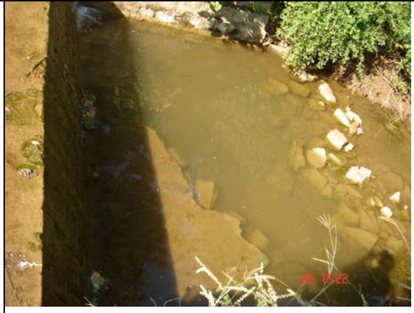
Picture 8. Damaged apron wall of the left side masonry check dam.
