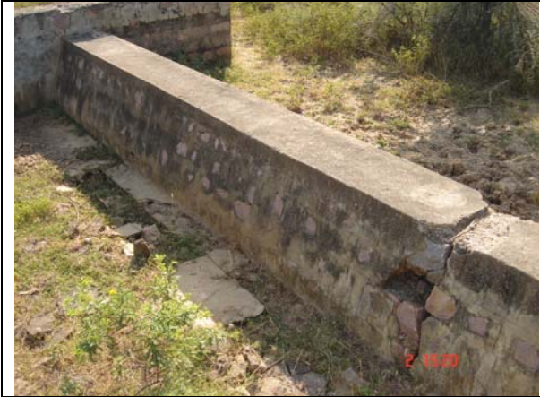
Picture 32. Damaged check dam in Sanjeevanraopet watershed serving no purpose.
