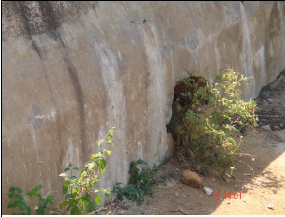
Picture 27. Leakages/damages on masonry check dam in Rayalamadugu watershed.
