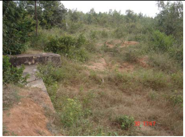
Picture 14. Condition of the masonry check dam constructed in forest land in Lakshmisagar watershed
