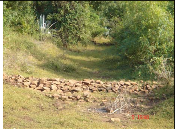
Picture 16. Condition of the damaged loose boulder structure in Maddikunta watershed.
