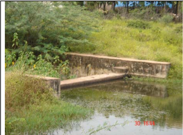
Picture 23. Masonry check dam in the Mudimanikyam village constructed for recharging the community bore well.
