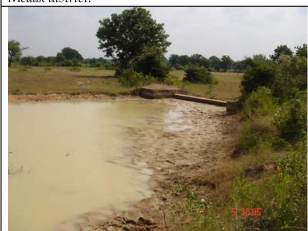
Picture 38. Masonry check dam with lot of silt accumulation in Siddapur village.
