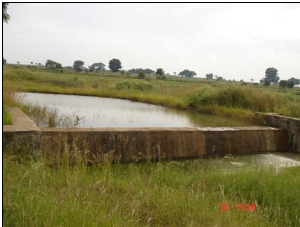
Picture 3. A masonry check dam with Good storage of water at Aksanpally
