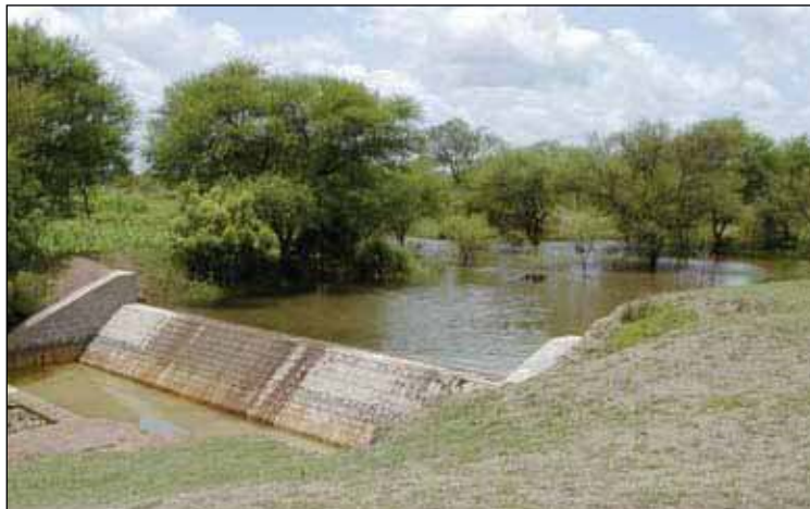
Figure 10. A masonry check dam at Kothapally watershed, Ranga Reddy, Andhra Pradesh.
