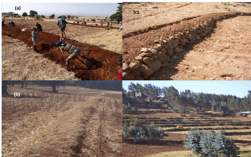
Fig. 2. Photos depicting soil and water conservation practices (SWCPs) in the study area: (a) Newly constructed soil bund in the Debre Mawi watershed (January 2014, photo by Dr. Gizaw Desta); (b) Stabilized soil bund in the Debre Mawi watershed (November 2023, photo by Aschalew Kassie); (c) Newly constructed stone bund in the Abaa Gerima watershed (January 2014, photo by Dr. Gizaw Desta); (d) Stabilized stone bund in the Abaa Gerima watershed (November 2023, photo by Aschalew Kassie).
