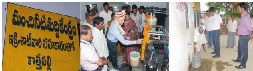
Fig. 11.3 RO plant in Kothapally village
