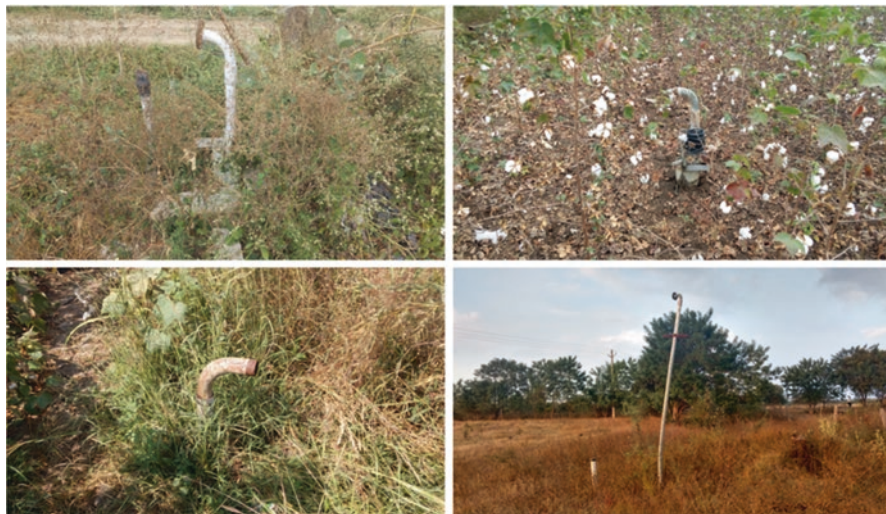
Fig. 8.27 Non-functioning borewells in Kothapally
