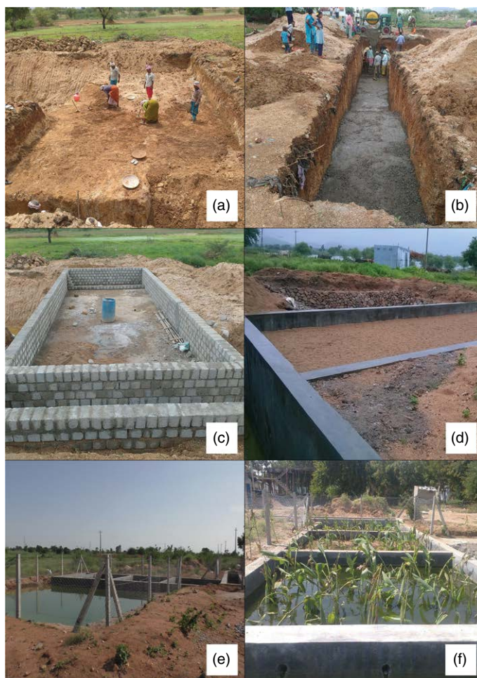
Fig. 12.3. Different phases of construction of the DWAT unit: (a) excavation; (b) concrete liner; (c) brick-masonry work; (d) plastering and curing; (e) fencing; (f) plantation.
