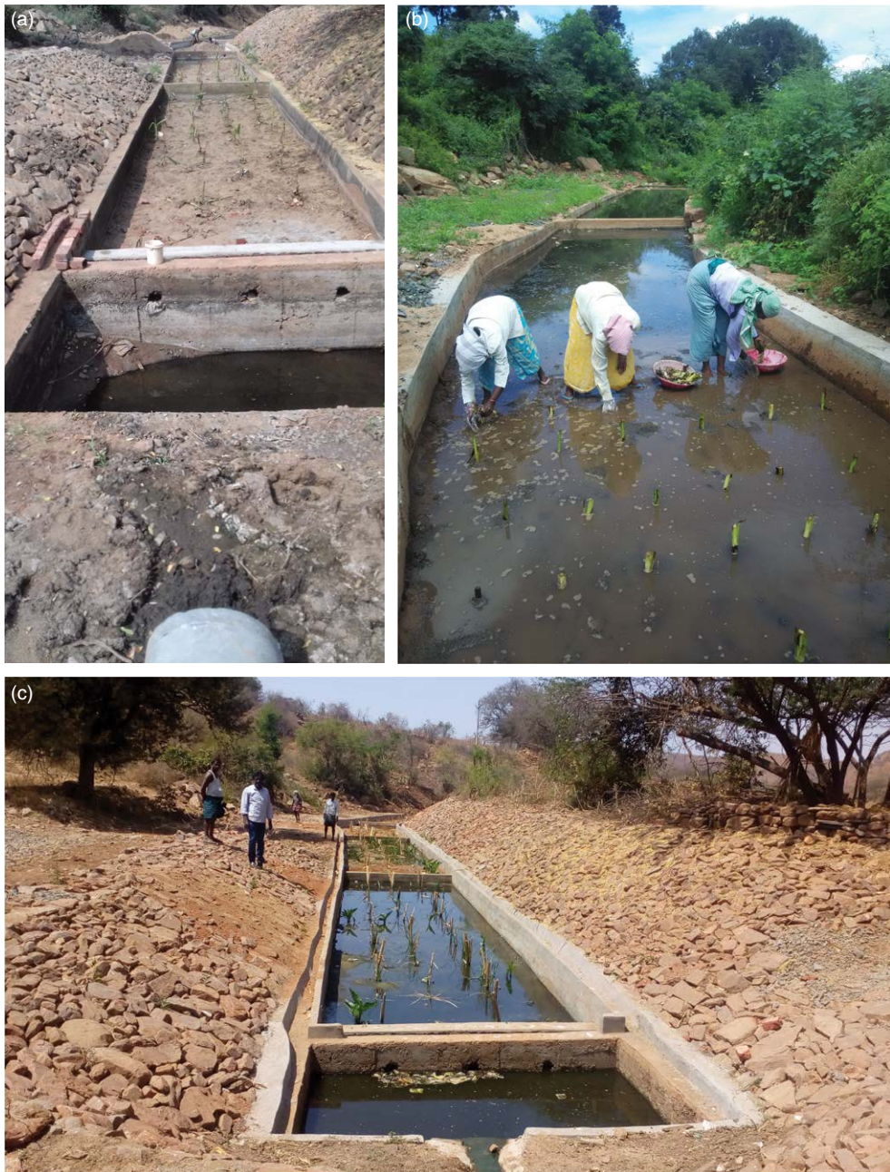
Fig. 10.5. Different phases in construction of decentralized wastewater treatment DWAT unit in Pendekal village: (a) construction of tanks; (b) planting of Canna indica ; (c) fully constructed DWAT unit during stabilization phase.
