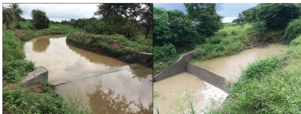
Fig. 6.5. Check-dam filled with water during the rainy season in September 2016 in Bhanoor village.
