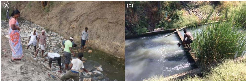
Fig. 6.6. Construction of wastewater treatment plant in Bhanoor village: (a) in progress; (b) completed structure.
